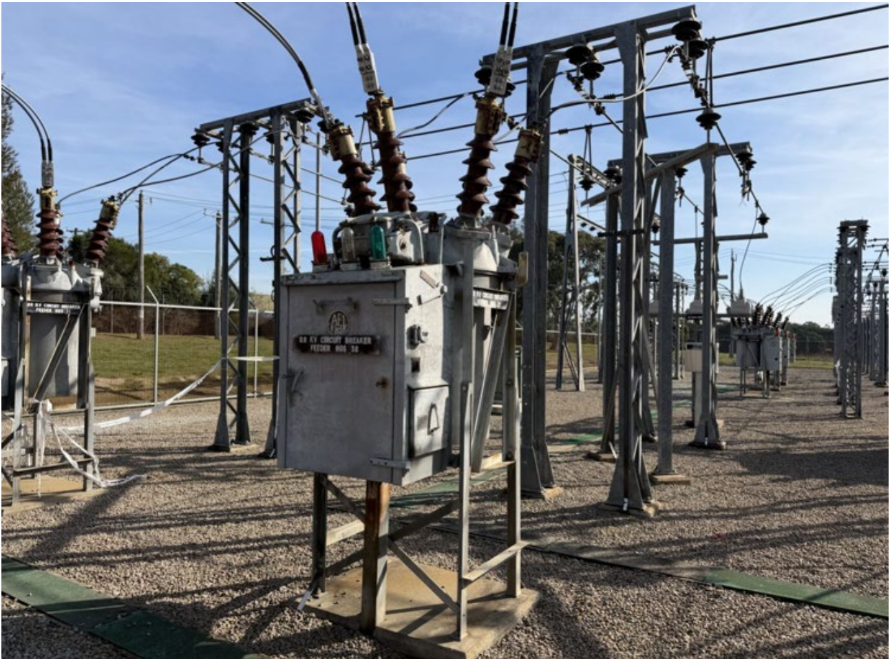
Figure 7: Existing outdoor 22 kV circuit breakers at HGS
