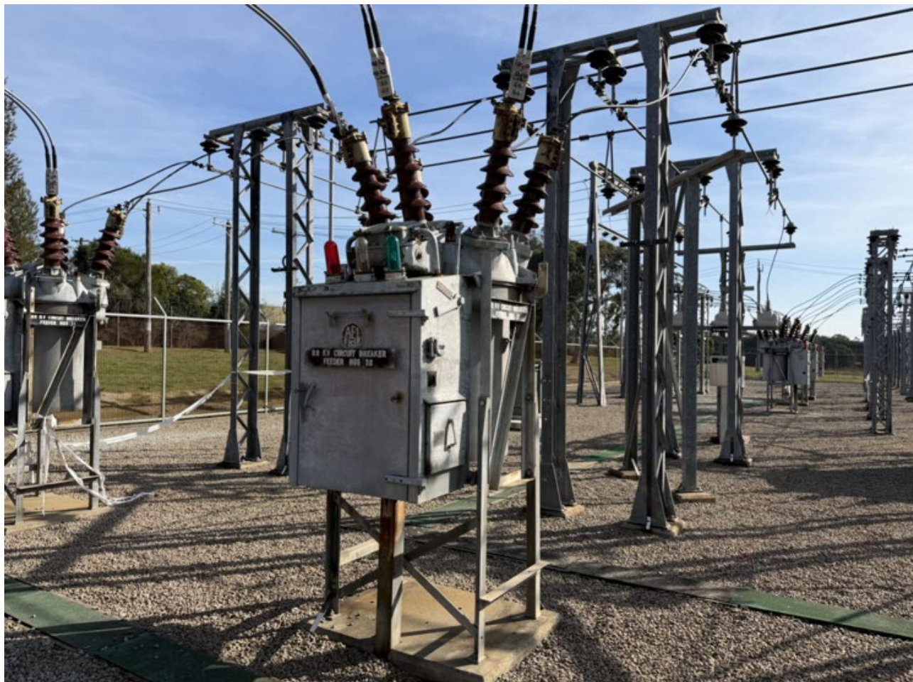
Figure 7: Existing outdoor 22 kV circuit breakers at HGS
